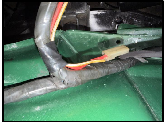
Loose coil wire
